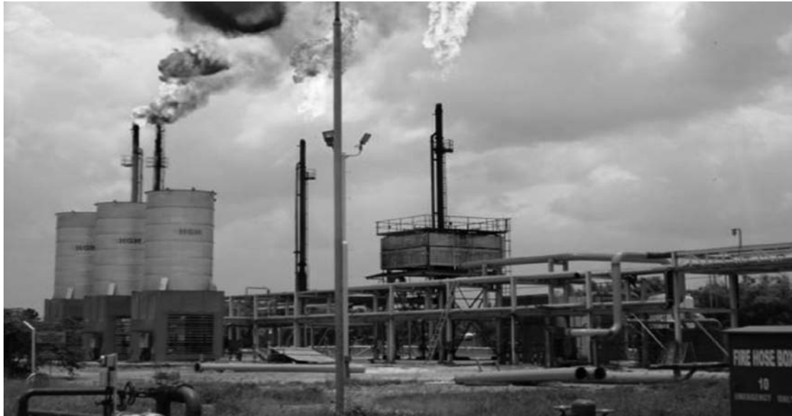
Flares and heat-sound exchangers at JOB PetroChina–Pertamina desulphurization unit.
