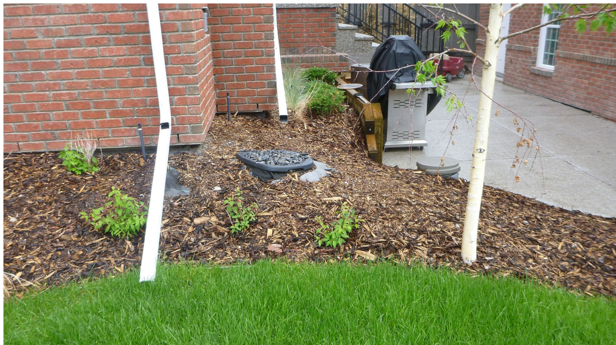
Figure 29. Rainwater harvesting and irrigation system in Calgary, Alberta
