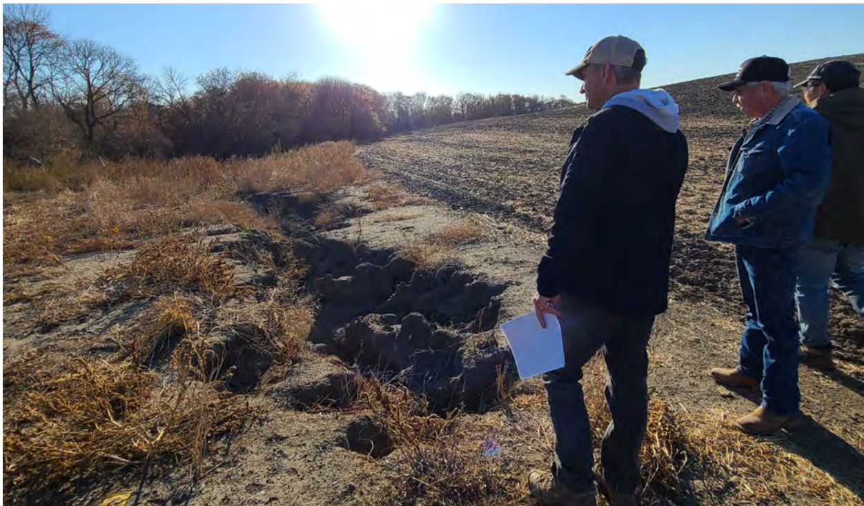
Figure 38. Newly discovered and incipient gully erosion downstream near a feasible critical area planting BMP site
